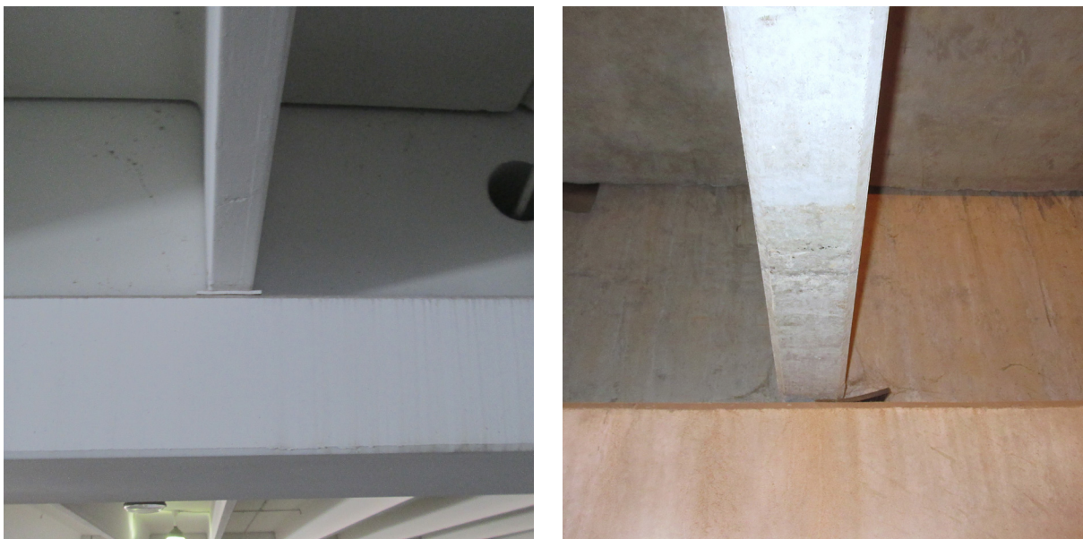
Figure 2.2. Proper double-tee bearing pad position on support surface reduces the potential for distress. The photo on the left shows a pad that is properly centered with respect to stem width. A misplaced or displaced pad (right photo) can cause spalling. Photos: Michael Lee.
