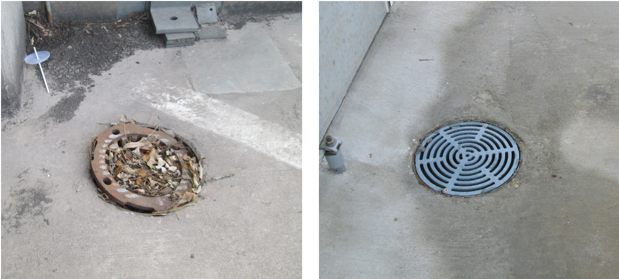
Figure 2.5. Comparison of a clogged and unclean floor drain (left) and a clean floor drain. A clean drain promotes surface drainage and therefore mitigates deterioration of concrete deck. Photos: Michael Lee.
