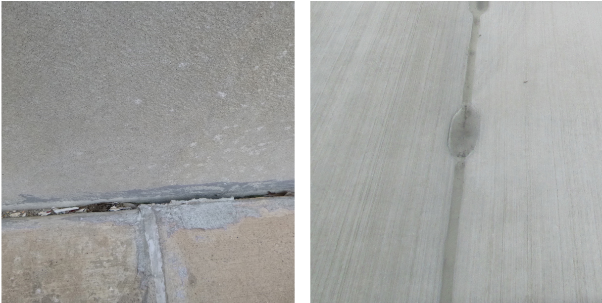
Figure 2.1. Housekeeping should include frequent cleaning of joints. The joint shown in the left photo contains debris. Clean joints (right photo) will increase service life. Photos: Michael Lee.
