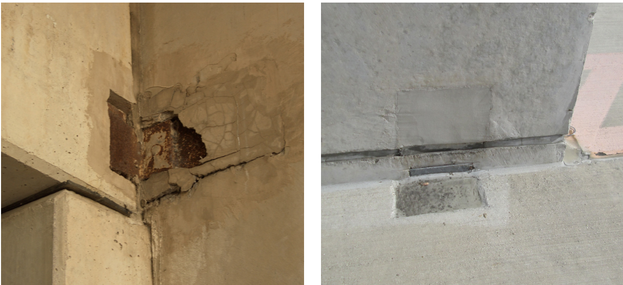
Figure 2.6. Comparison of a recessed connection exhibiting cracking along perimeter and spalling of grout cover (left) and a grouted connection in excellent condition. Photos: Michael Lee.
