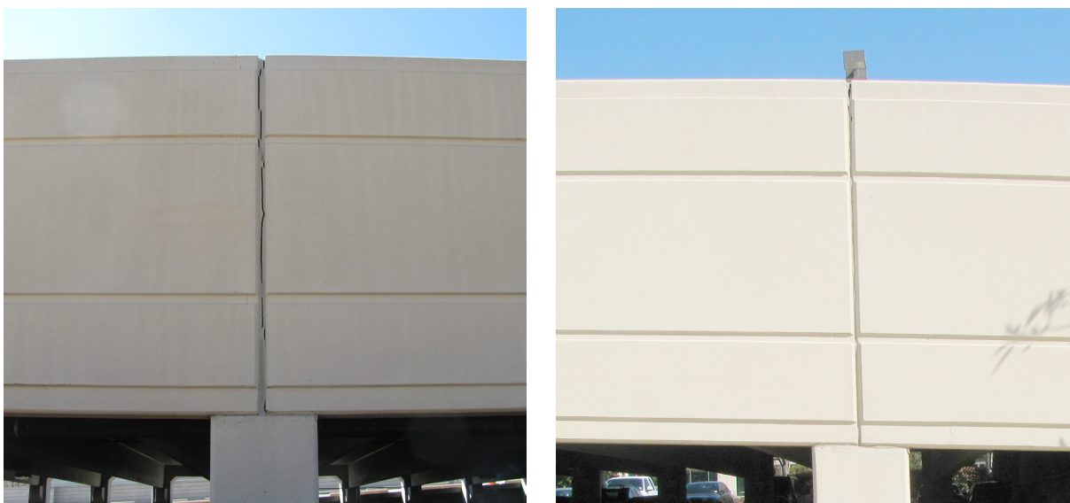
Figure 2.7. Comparison of debonded and torn joint sealant (left) and sealant in good condition. Photos: Michael Lee.
