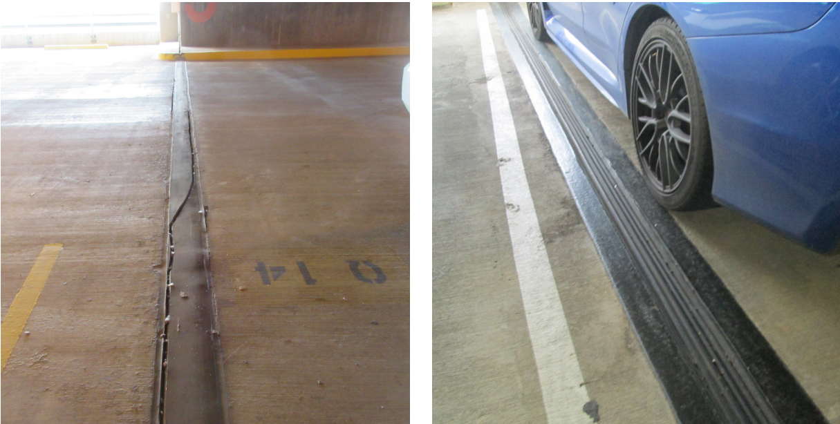
Figure 2.4. Comparison of a debonded and torn expansion joint seal (left) and a seal in excellent condition. Photos: Michael Lee.
