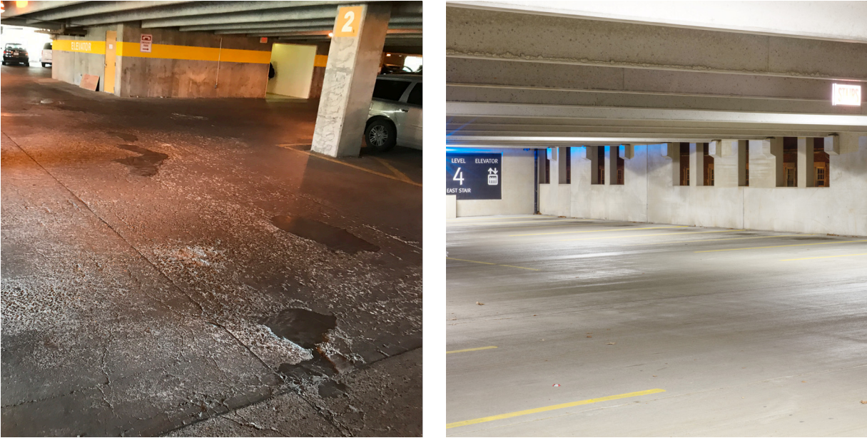
Figure 2.3. Comparison of a deck surface exhibiting excessive deterioration (left) and a deck surface in pristine condition. Left Photo: Michael L. Lee. Right Photo: Ted O'Shea.
